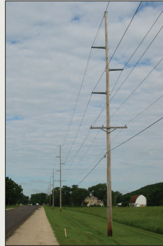
69-kV/115-kV transmission structure with distribution underbuild
