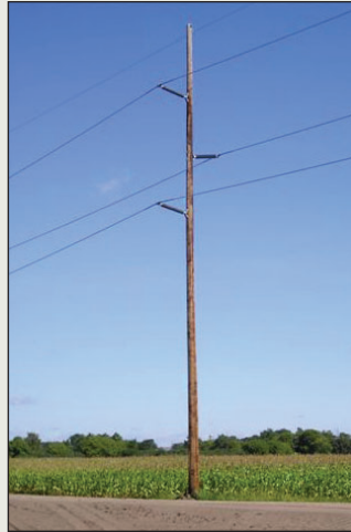
69-kV/115-kV transmission structure
