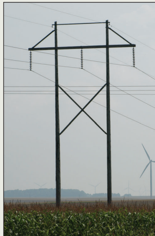
230-kV/345-kV H-frame transmission structure
